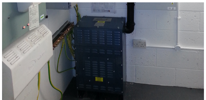
The Powerstar unit installed at the Centre.
