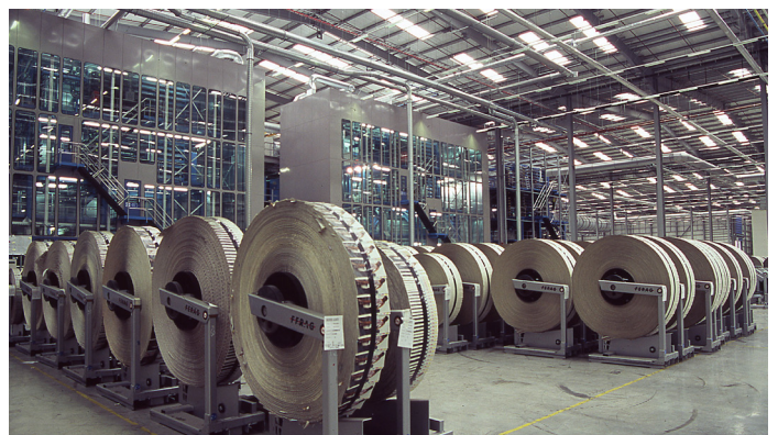
Powerstar reduced harmonics on site.
