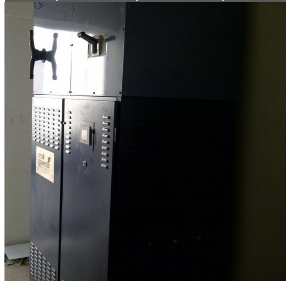
The Powerstar installation in the Papantoniou store.
