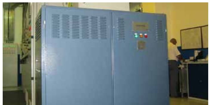
Powerstar installation at Ski Dubai.
